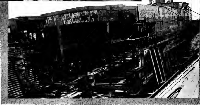
The two lower pictures show the character of one of the largest ship surgery jobs yet carried out. The after end of the steamer "Moreland" is shown under reconstruction at Superior, Wisconsin, July 21, 1916, and the open ends of the two sections are also shown in drydock on September 16, 1916.
